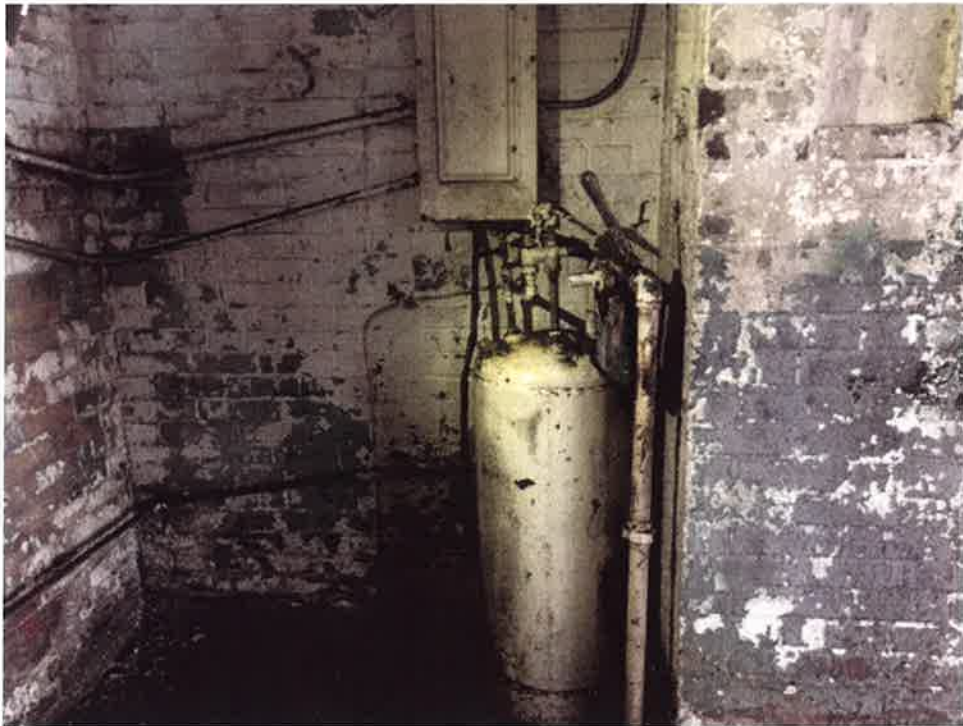
Photo No. 10 Description Air compressor tank inside garage bay #1 Date December 23, 2015 Photographer S. Pfeifer
