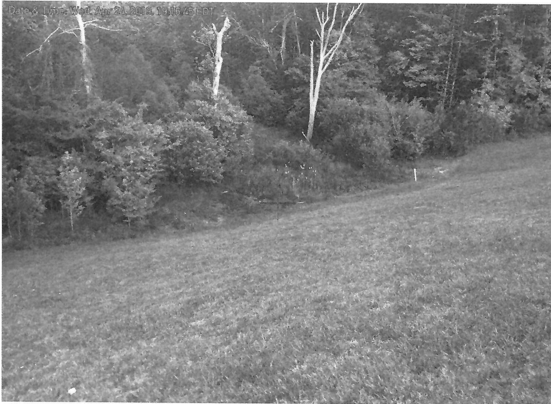
View from downstream edge of crest at Main Dam. Standing water at toe of slope.
