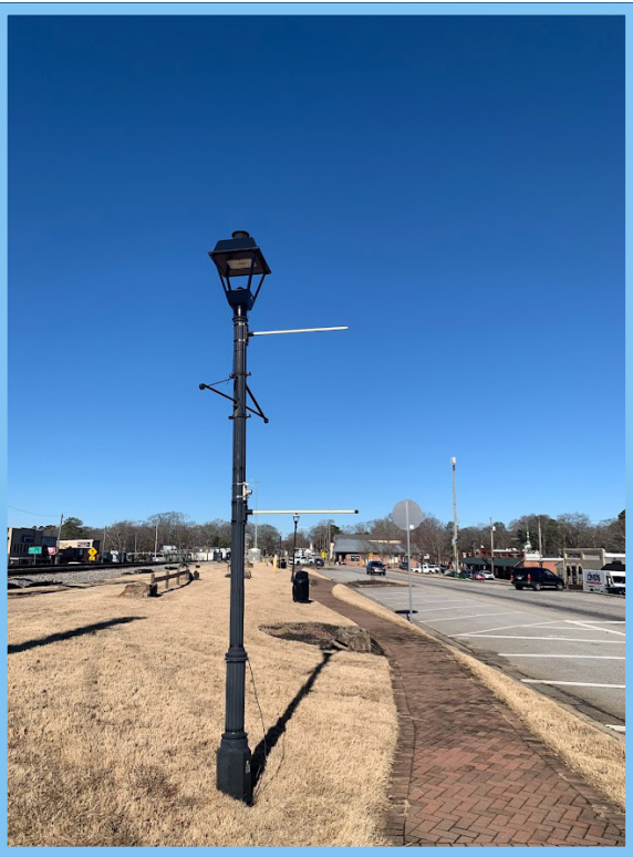
Freestanding Luminaire on Post
