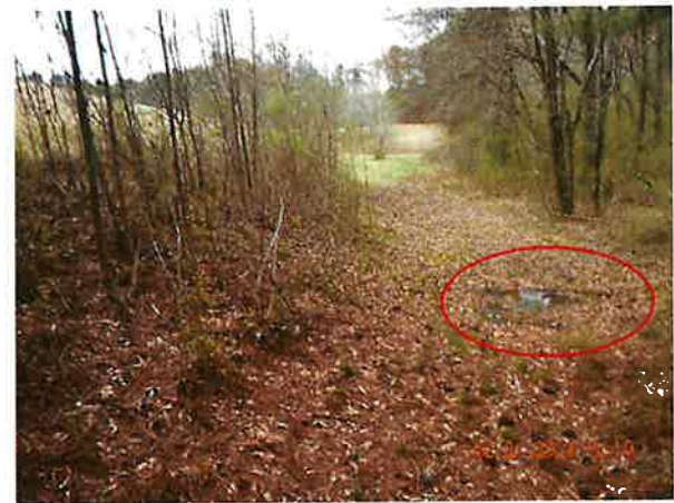
Trees on the right downstream slope and encroaching on the slope with wet/saturated area and standing water between
