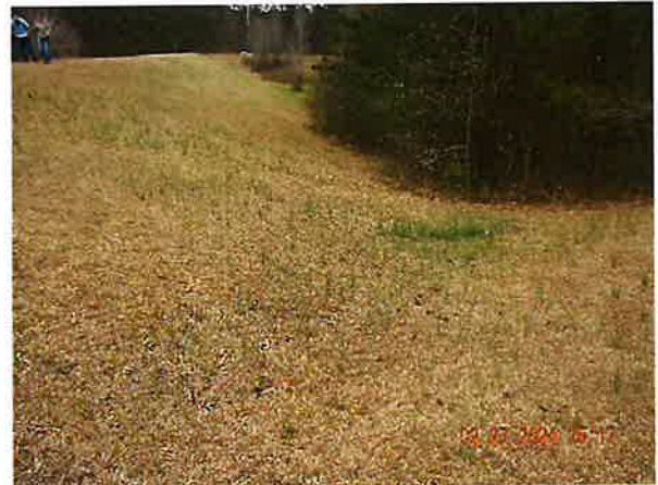
Looking left from right abutment at trees encroaching on the right downstream slope
