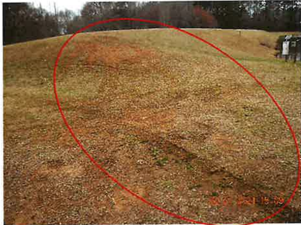
Bare and thinly grassed areas from the left auxiliary spillway onto the crest
