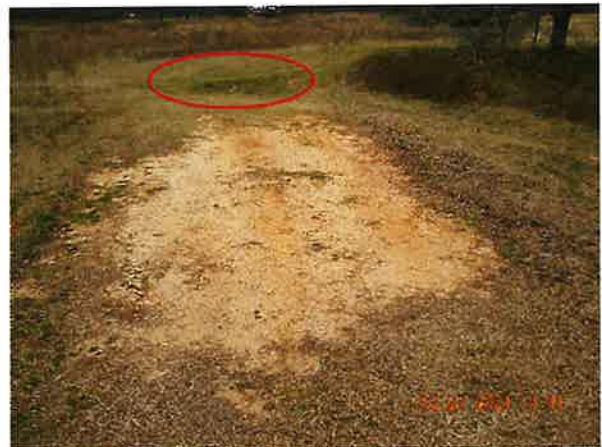
Looking right from right crest with erosion into the auxiliary spillway; wet area with standing water circled
