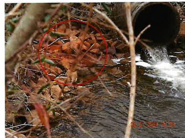
Overgrown plunge pool and orange staining with flow in area of likely buried right drain
