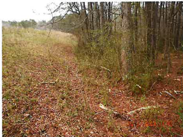
Looking left on right downstream slope at trees and brush encroaching
