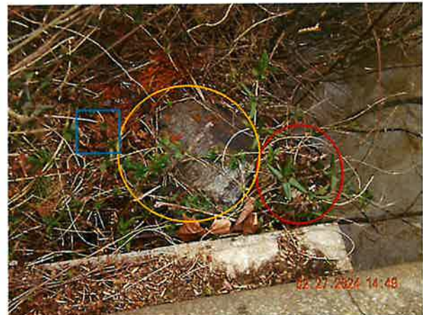
Looking left at top of left drain outlet, large rock, and stump
