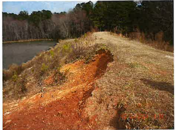
Gully on upstream slope near the principal spillway encroaching into the crest
