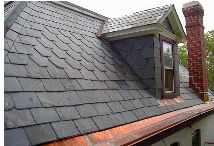
An example of a poor replacement of slate shingles that is not “in-kind” with the original shingles. All shingles should be the same shape in this example.
